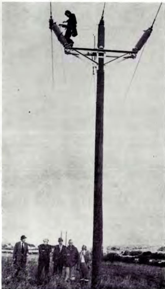
Inside a safety rope enclosure, the linesman demonstrates the ease of working on the line end of one of the outside insulators. Below, without crash helmets as this was a posed-for picture, are Messrs. Mike Hughes, Arthur Perry (Asst. Chief Engineer, Construction), Des Wallin (Murphy's), Ken Jones and Geoff Price.
